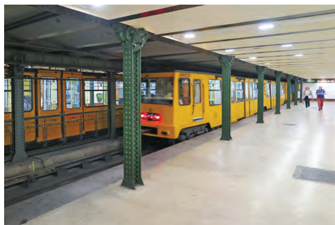
Platform of the historic line M1 or földalatti railway. Note the decorative cast iron capitals on top of the girder roof supports
